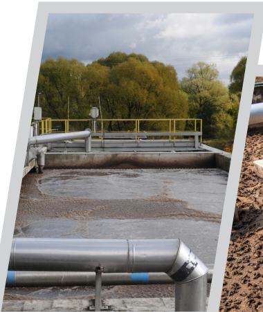
BACK WASH RECOVERY TANK
