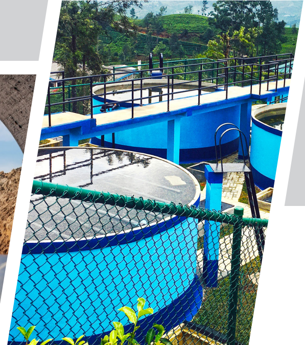
PACKAGE TREATMENT PLANT
