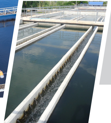
RAPID SAND FILTER & GAC FILTERS
