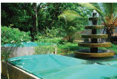
Ensuring a clean environment - the water treatment plant at our Siyambalape facility
